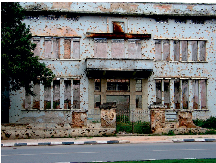
Building in Huambo showing the effects of war. Image: Wikipedia
